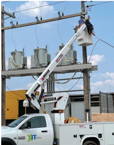
An XIT crew member is pictured above working on a customer's aerial fiber.
